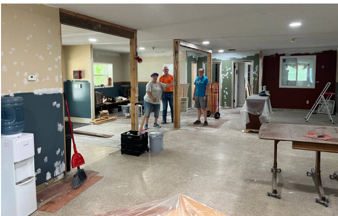
Scott Hilburn, Robin Traffas and Katy Nininger hard at work on the renovation project.
